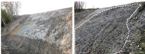
Fig. 3. Man-made slope in Øysand site before (left, November 2019) and after failure (right, April 2020)
